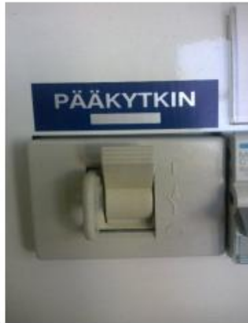
Main switch in the I position.
