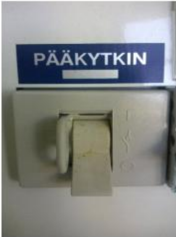
Main switch in the 0 position.
